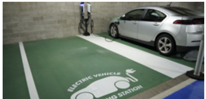
Arch Garage, Electric Vehicle Charging Station
