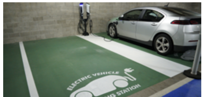
Arch Garage, Electric Vehicle Charging Station
