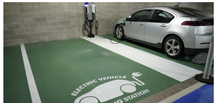
Main Parking Garage, Electric Vehicle Charging Station
