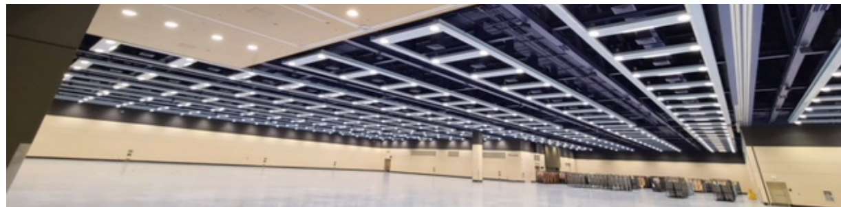
The Center converted over 1,000 bulbs from metal halide to LED in exhibit halls and the Skybridge, saving energy and lowering expenses.
